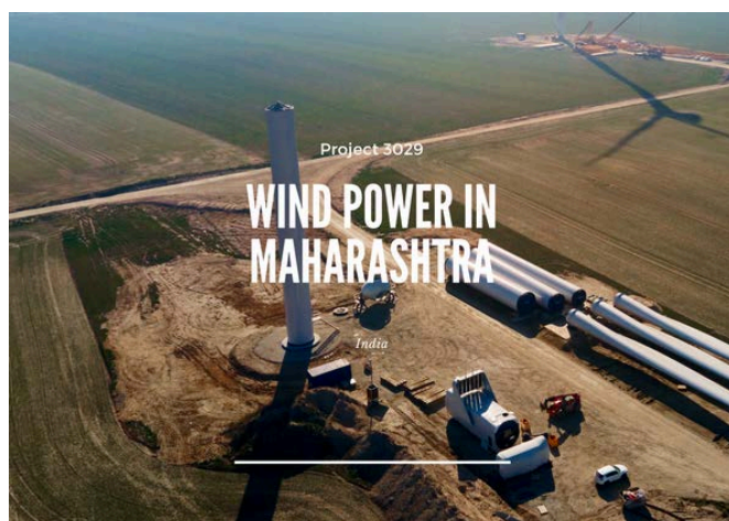
Project 3029: Wind Power in Maharashtra
